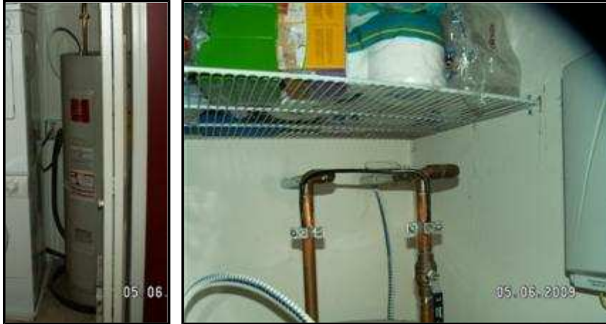
Water Cut Off Valves
